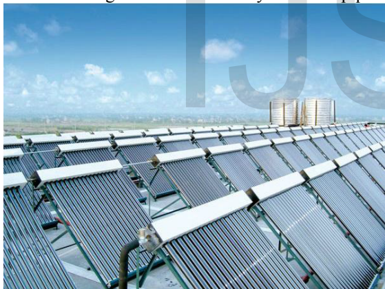
Fig3. Shows Solar Water Heating System
